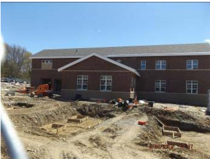
Photo depicts the progress of the exterior along with progress of the carport footings
